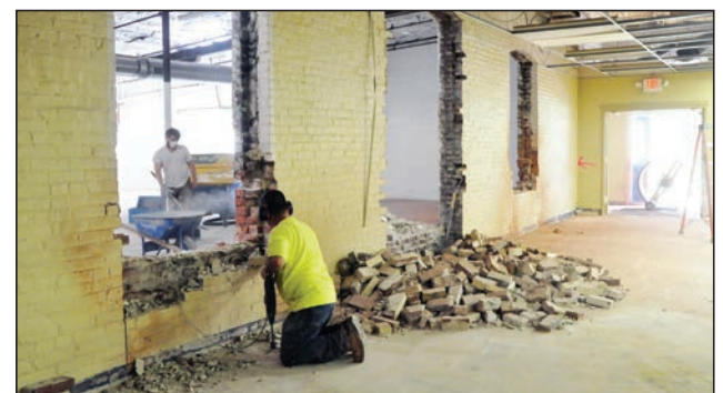
A worker for Stenz Construction removes bricks from a covered former window on June 15 inside the distribution center of the St. Vincent de Paul Indianapolis Council in preparation for the opening of the council's thrift store, Mission 27 Resale, in October.
